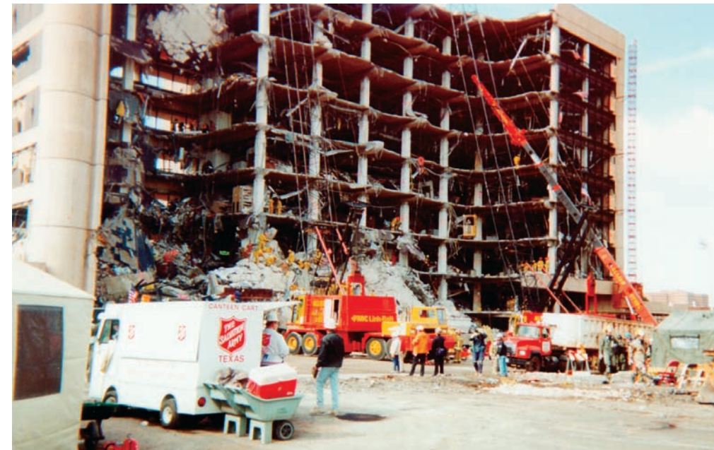
Alfred P. Murrah Federal Building, April 1995 Oklahoma City, OK
